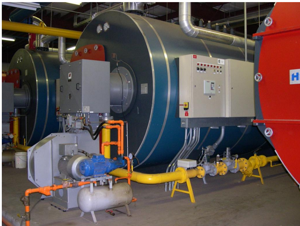
Figure 2. Central heating system with boilers located outside the greenhouse.
