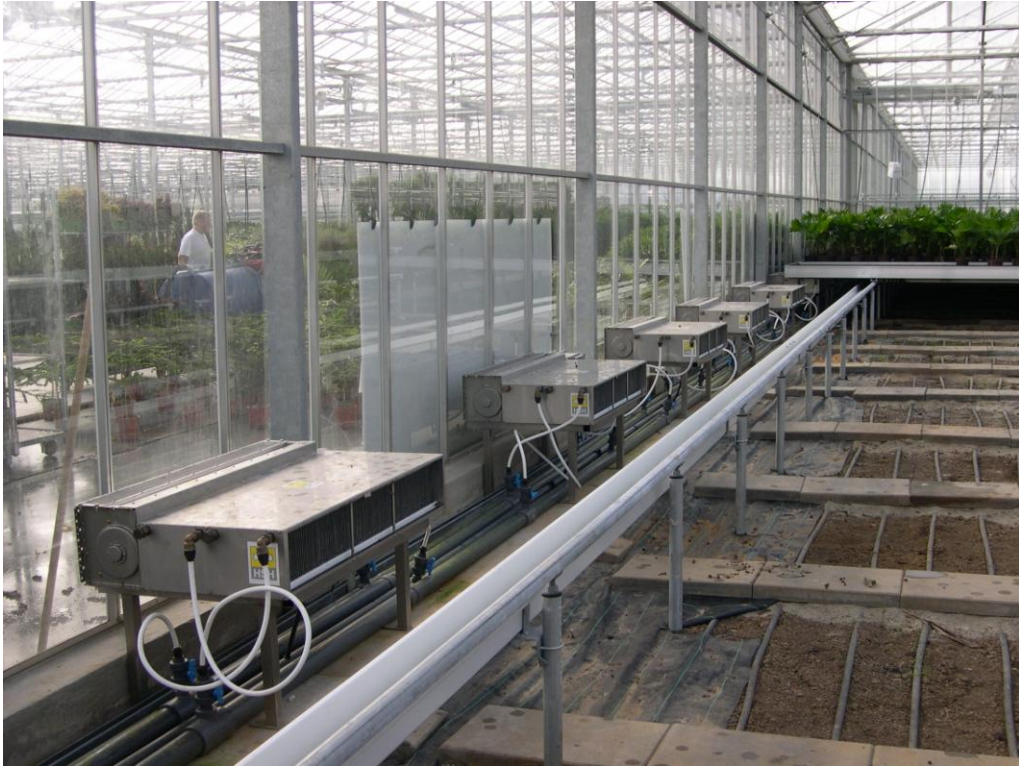
Figure 4. Efficient heat exchangers to collect heat from the greenhouse air during summer. The heat is stored in the aquifer.
