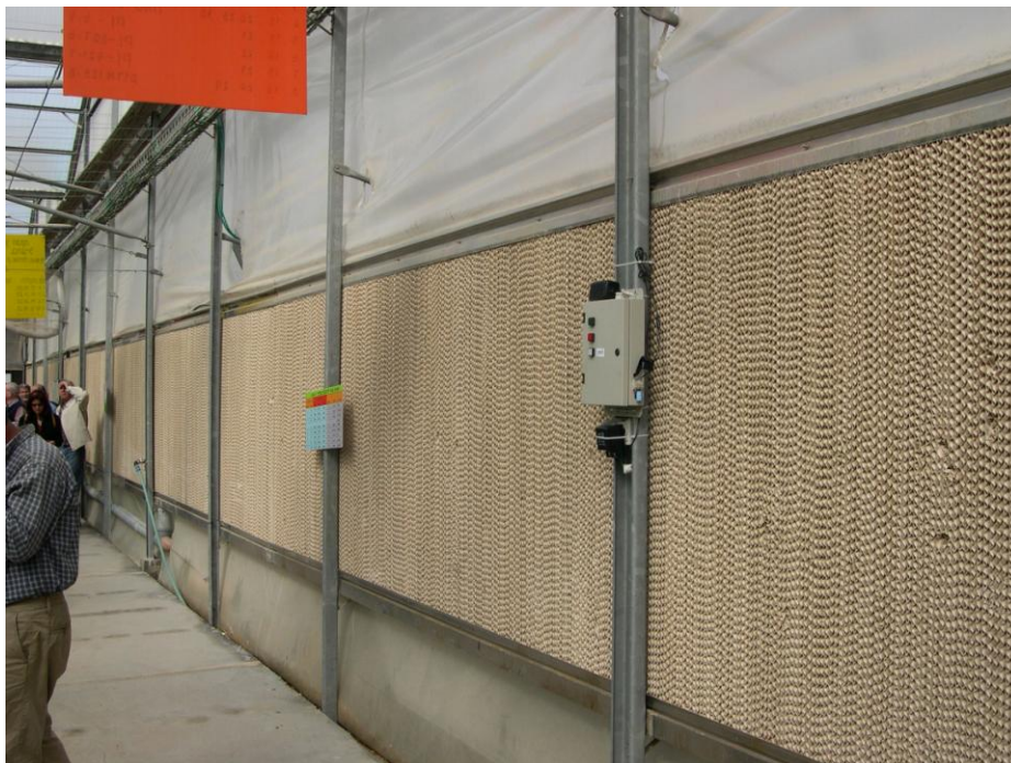
Figure 6. Vertical pad in a greenhouse cooling system.
