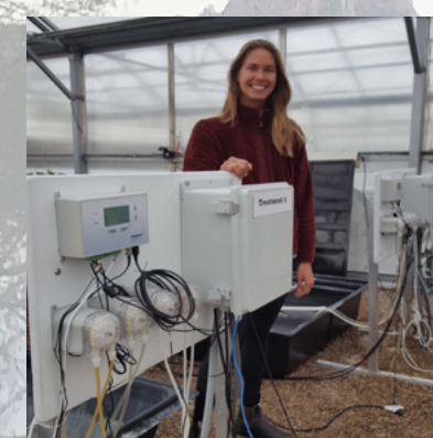
Allie Allgeyer with fertigation controls from Autogrow, Inc.
